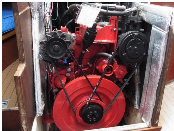
Rapture's Engine Room
