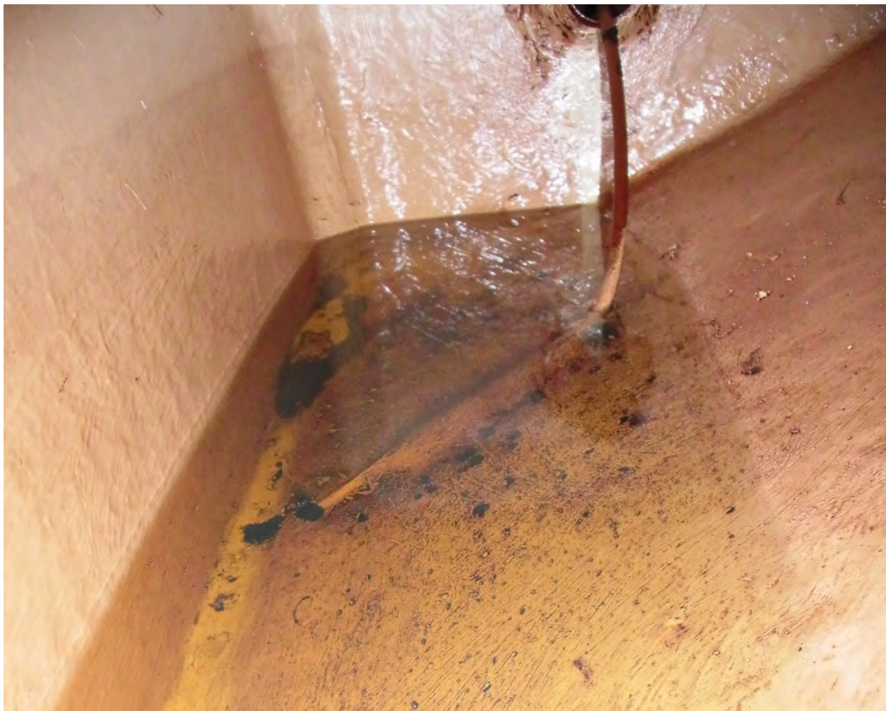
Inside Tank Before Cleaning Note dirt at mouth of Fuel Intake
